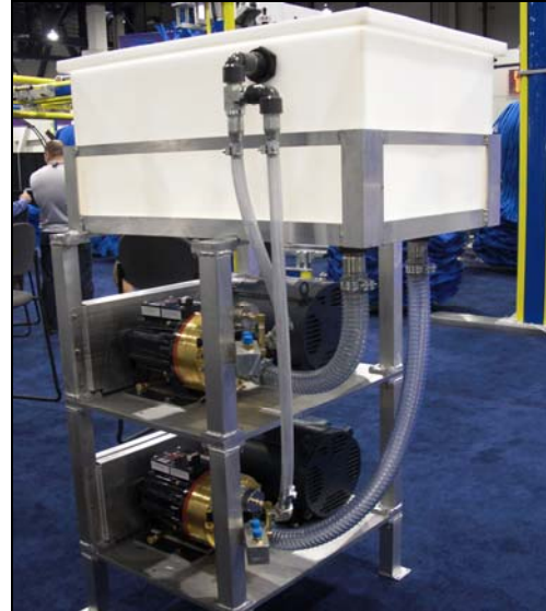
Pic #2: Dual 15HP Pumping Station
