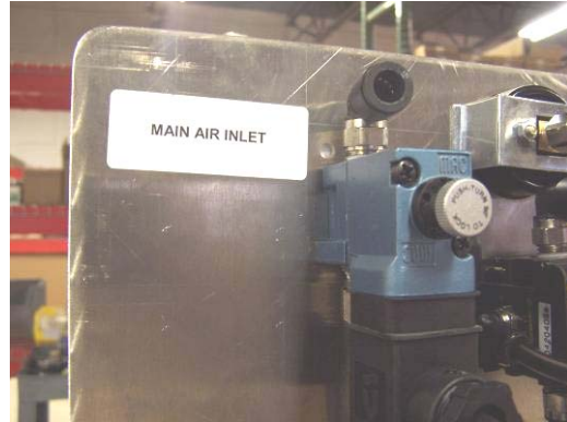
Pic #5: Solenoid valve Air Inlet
